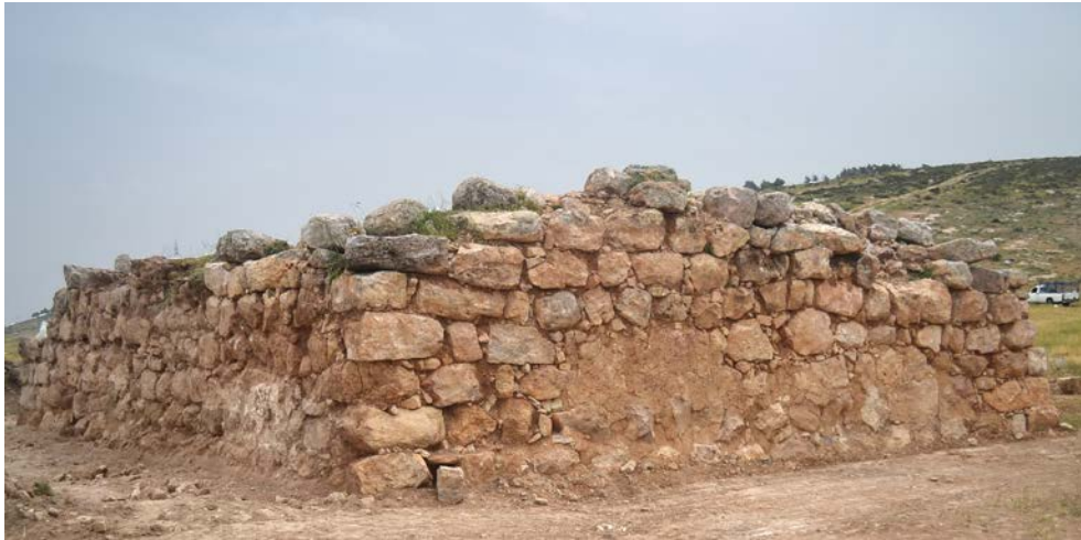
Fig. 9 - The NW corner of the podium with preserved original plaster; from the north-west.
