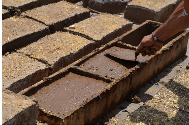
Fig. 15 - Making of mud bricks to be used in the restoration of Palace G.
